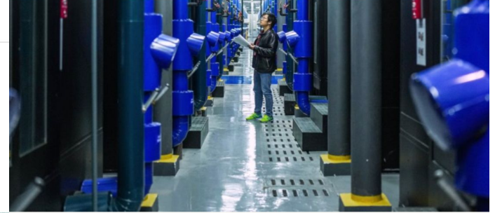
Center of China Unicom, which uses artificial intelligence in its operations. TAO LIANG / XINHUA VIA GETTY IMAGE
